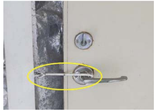
Hold back hook - Unacceptable
