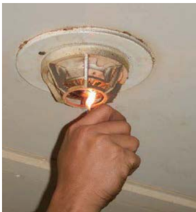
Improper test method
