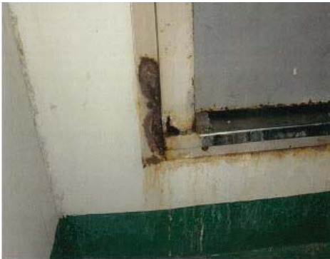
Worn out and wasted fire door frame
