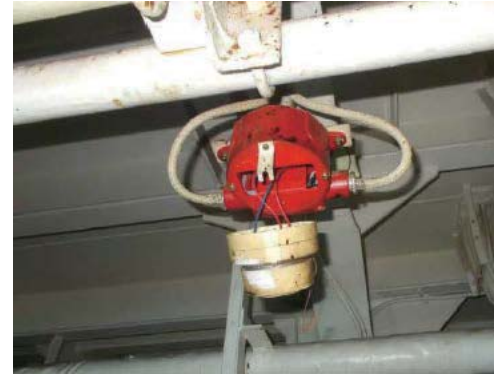
Defective fire detector
