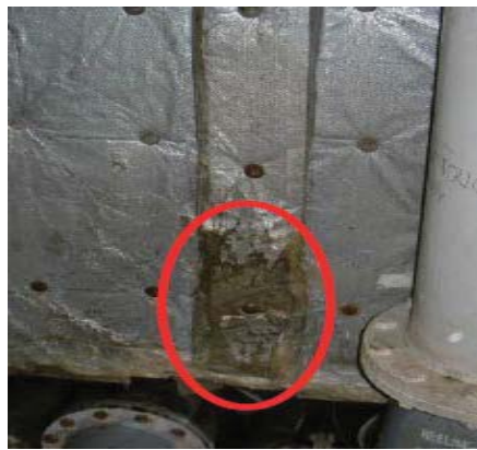
Partly missing Class A insulation
