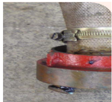
Fire hose end secured using unapproved method
