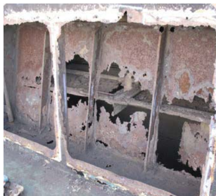
Fire damper wastage found after removing cover
