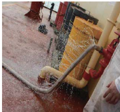
Leaking fire hoses
