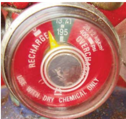
Fire extinguisher not charged
