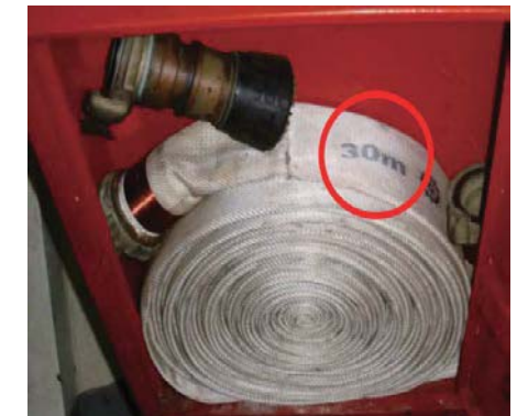
Length of fire hose in Engine room more than 15 M
