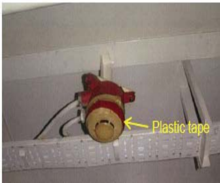
Fire detector covered with plastic tape
