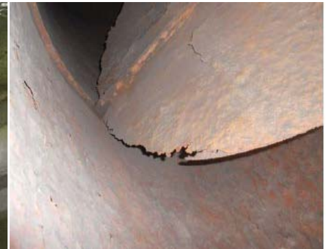
Fire damper flap wasted
