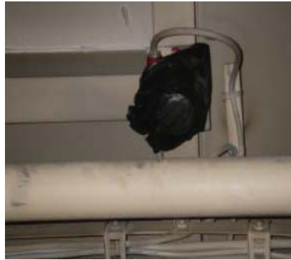
Smoke detector covered with plastic bag
