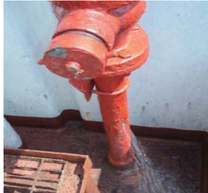
Leaking fire line
